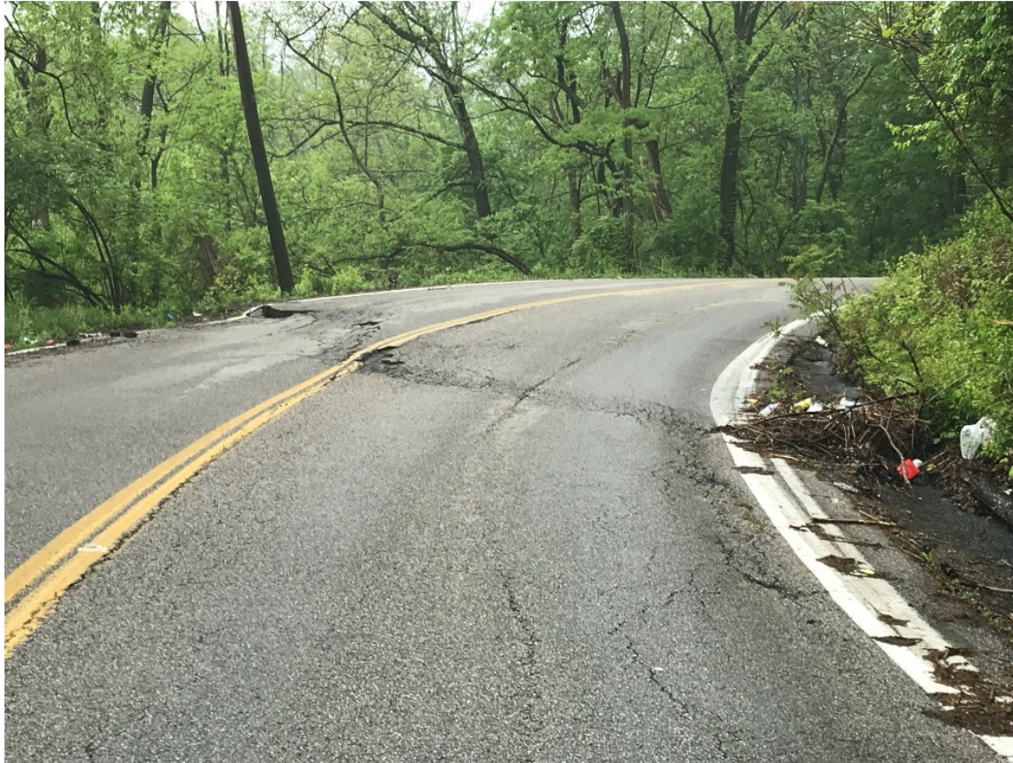
Faraday Road - Scarp (set down) in Pavement (has since been patched)
