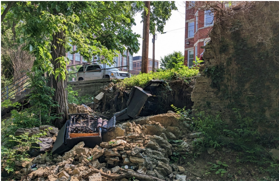
Eleanor Place - Collapsed Wall Section
