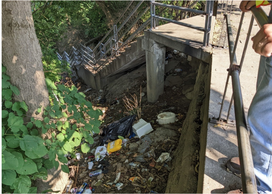
Eleanor Place - Upper Flight of Stairs (pushed by wall deflection)
