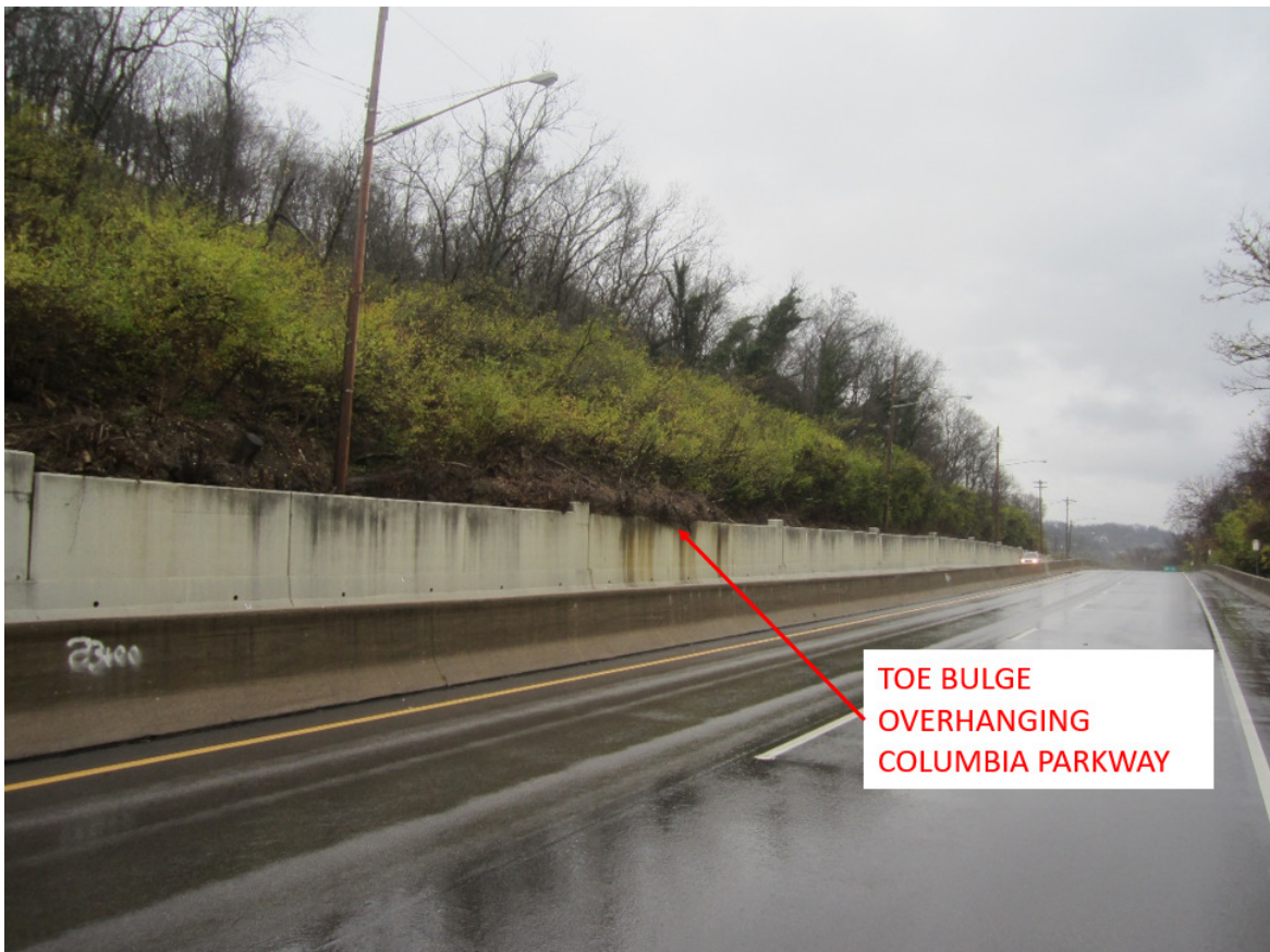
Columbia Parkway Landslide, South of Beechmont
