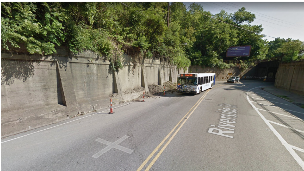
Riverside Drive at Rookwood Overpass Landslide
