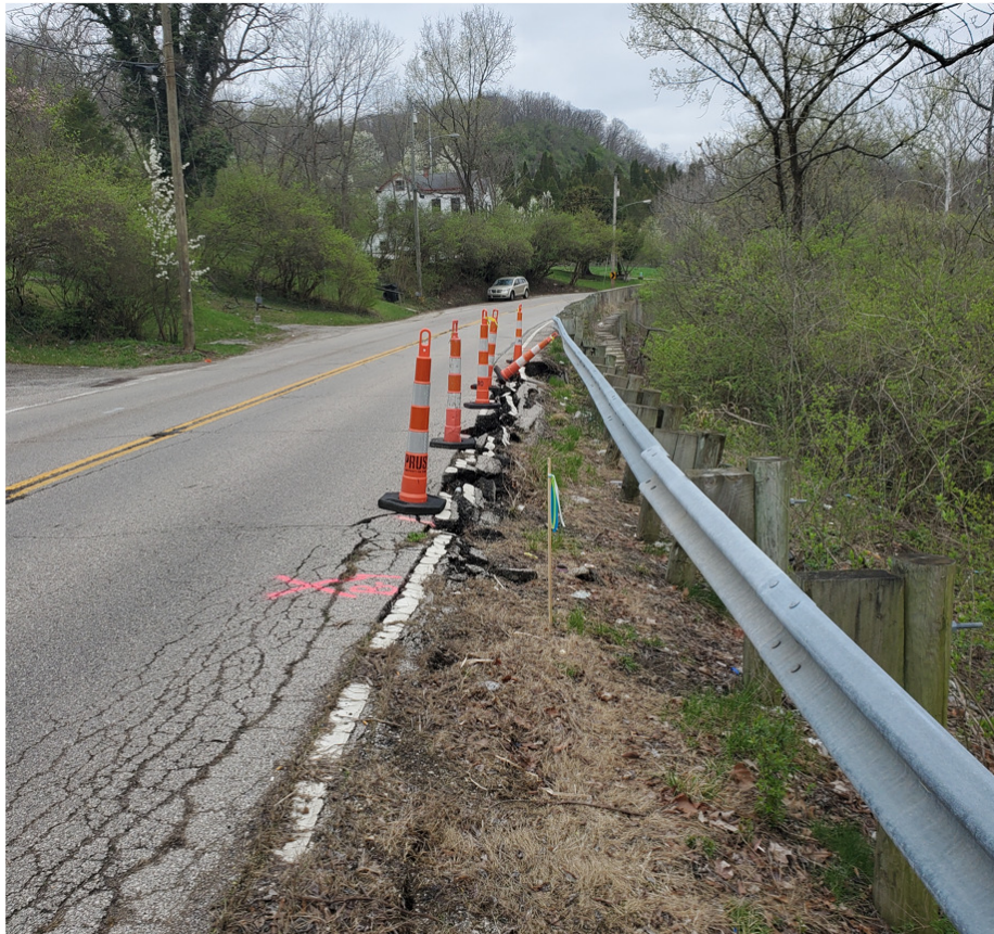
West Fork Road Landslide Correction, Before
