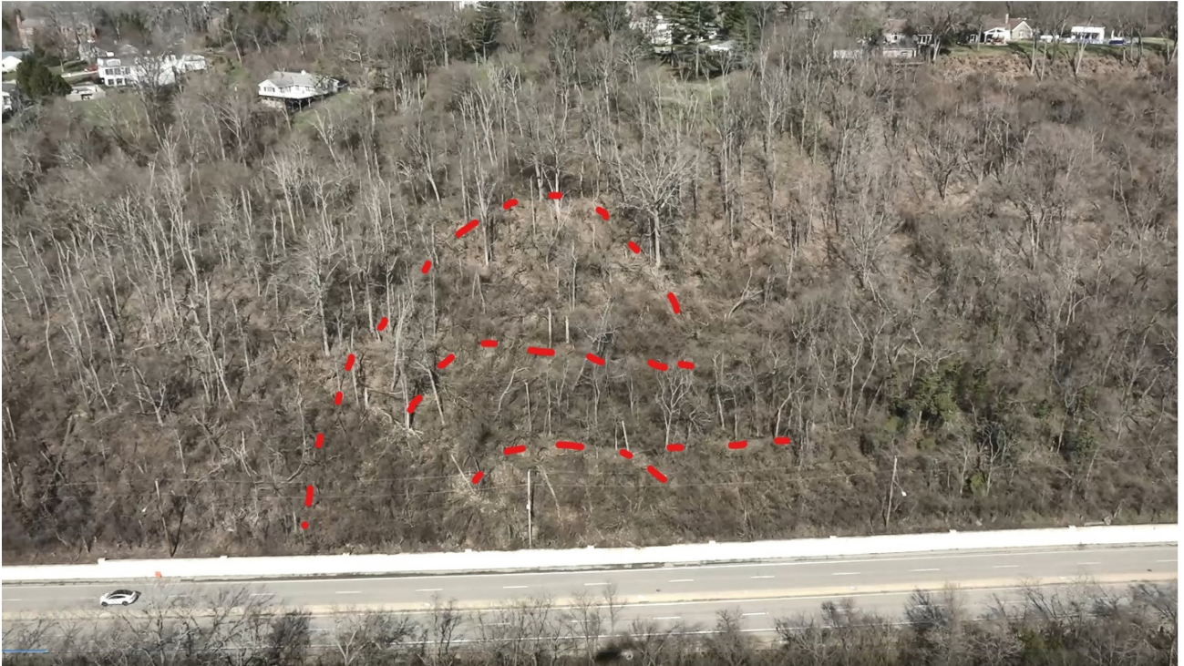
Columbia Parkway Landslide, South of Beechmont
