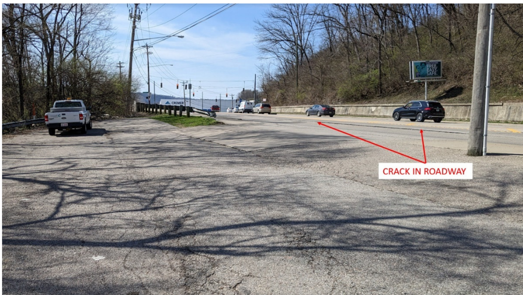
River Road (US 50) Landslide - East of Southside Avenue
